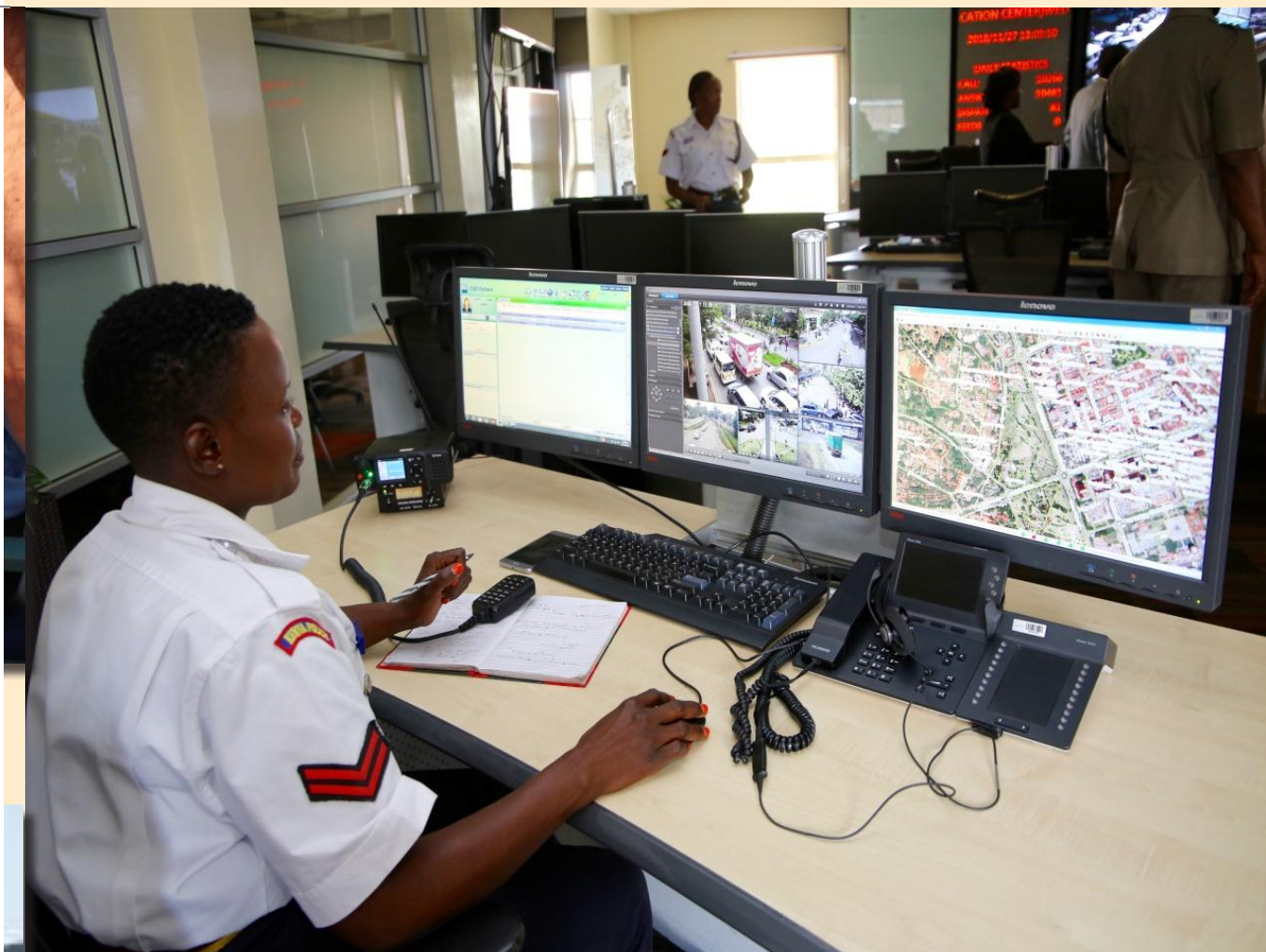
Integrated, Communication, Command and Control ( IC3 ) Centre.
