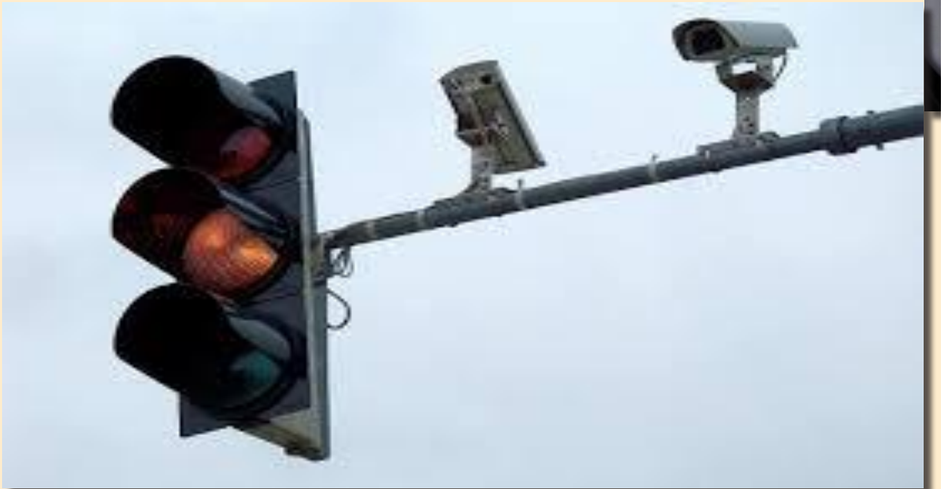
CCTV Cameras Installed in major cities across the country.
